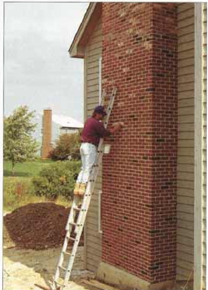
"Masonry artists" apply water-based, multipolymer stain and create the desired color blend.
