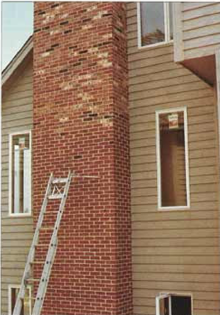
Too few range brick were delivered and installed, resulting in an uneven and unacceptable appearance.
